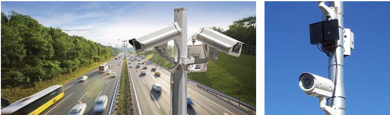
Closed-Circuit Television (CCTV)
